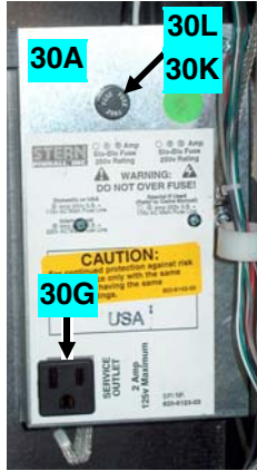
Enlarged Inside Cabinet View of Items 30: Power Box (30A), Service Outlet (30G), Fuse (30K) and Fuse Holder (30L).
